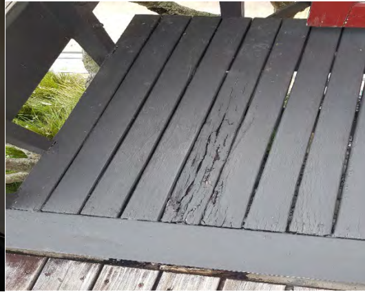
Image 5: 2 nd floor fire egress platform dry rot
