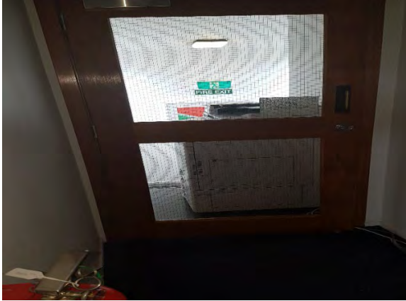
Image 4: Blocked fire egress
